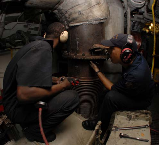
MK3 Jeffery and MK3 Gogo work diligently to reassemble the exhaust duct on the #2 Main Diesel Engine
