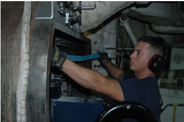
MK3 Rodriguez replaces the gaskets on the front cover of the boiler after "Punching the Tubes"
