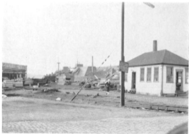
See that TR pacing along the Horn track? Pier 1 South Boston is already half demolished. What a fire those tinder timbers would have made. That was a good warm lonely shack, though.
