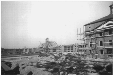
Construction of Liggett Hall or Building 400. The massive building was completed in 1880. Popular rumor was that it was built to prevent New York City from leasing the island and making it a municipal airport. The building stretches almost completely across the island.
