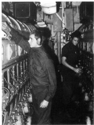
A clean engine room, is a happy engine room!
