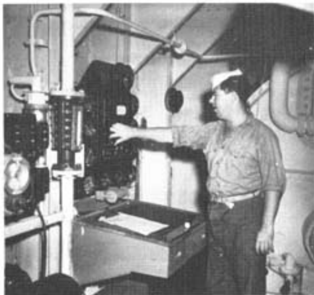
NO. 2 EVAPORATOR BOARD
