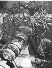
Generator that exploded
